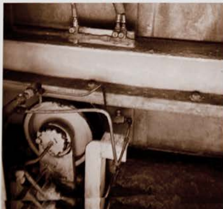
Lincoln Mist-O-Matic unit, shown below, spray lubricates rotating ring gear around perimeter of each filter.
